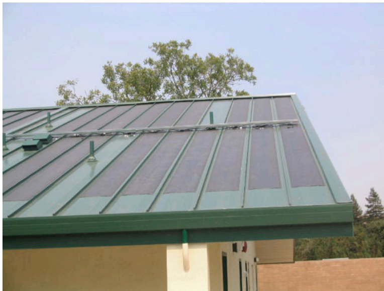
Self-adhering thin-film laminates installed over Garland's R-Mer® Loc standing seam roof system
