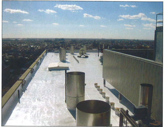
Introduced in the 1970s, polyurethane and polyisocyanurate products have helped revolutionize roofing. The material has become one of the most popular insulation components for U.S. projects.
