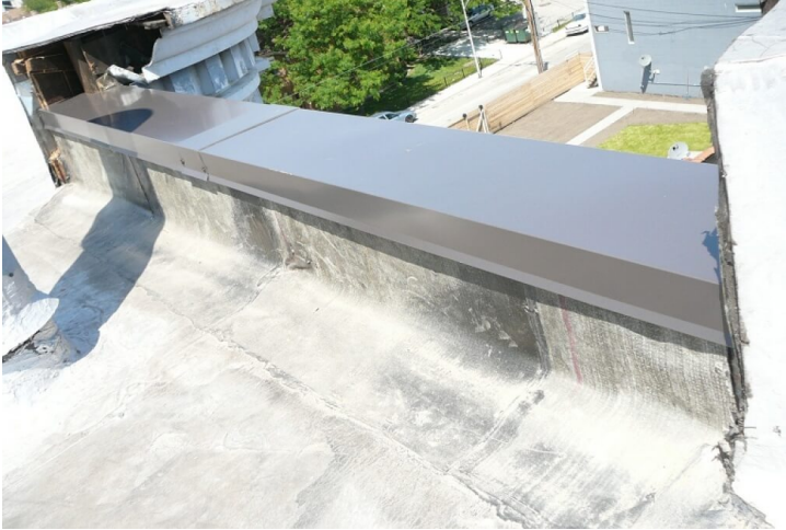
(Figure 2 A thorough roof investigation requires investigation of flashings for cracks.)
